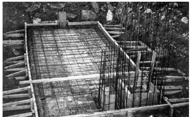
The top of the monitoring room being reconstructed in 1980. The turrets have just been started
